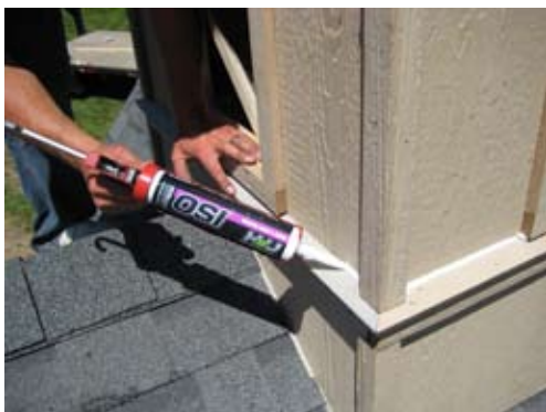
Run a bead of chaulking on all places where water can get to.
