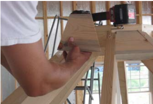
59. After all rafters are installed and fastened, fill in blocks that are cut on angles in between rafters.
