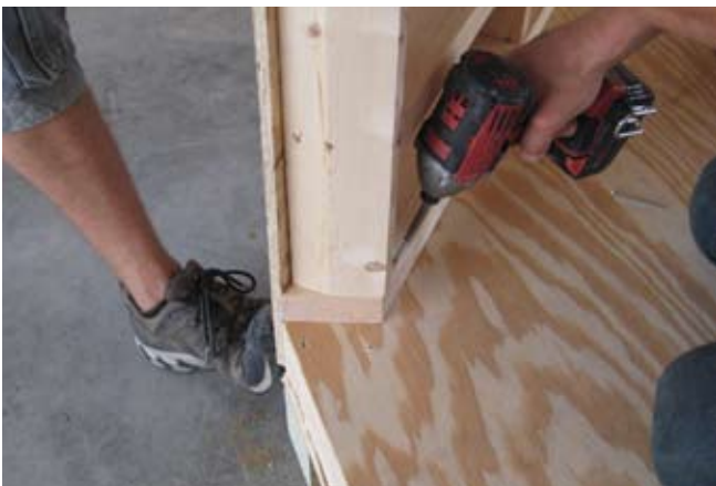
23. Secure wall panel A with 2 1/2" screws as shown. make sure corners line up and put pressure on the outside pushing in so wall is tight against floor as shown.
