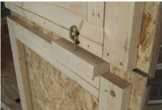
35. Barrel bolt is installed and 3/16" hole is drilled. This is what it looks like when completed.
